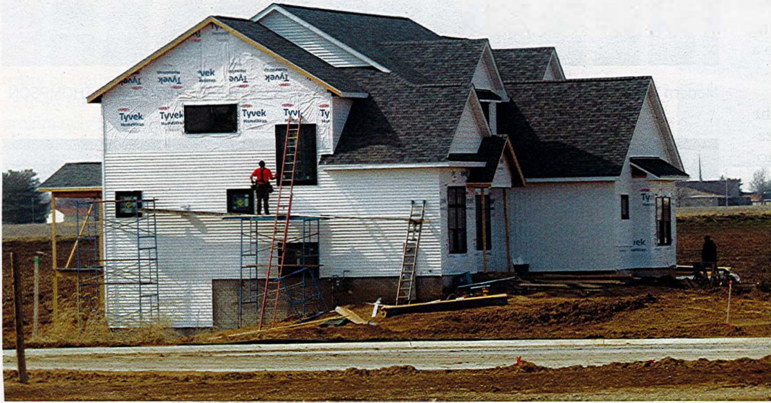
Work continues on a new home under construction off Hopewell Avenue in Bettendorf. CREDIT DAVE THOMPSON
